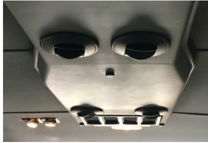
High-capacity roof mounted AC
